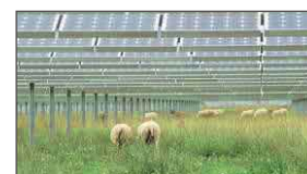
Farm solar generation system
